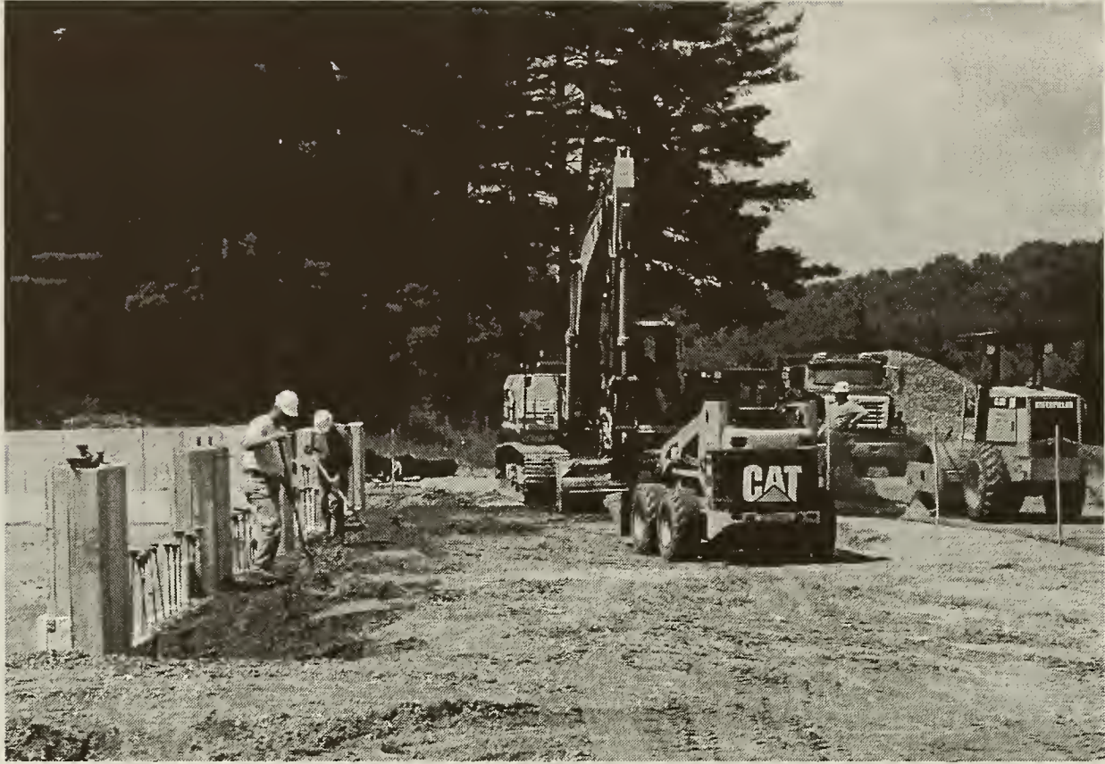
August 4, 2004. Backfilling by Derby Mountain Construction of Lyme, NH (assisted by the Lyme Highway Department).
